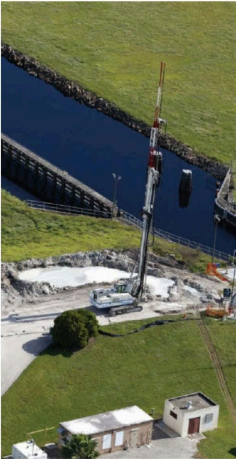
Above and previous pages: aerial views of the jobsite at Herbert Hoover Dike
